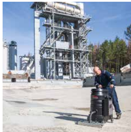
R01 D with floor suction device in asphalt mixing plant
